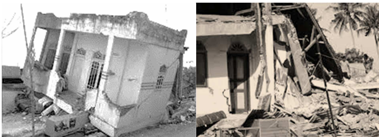
Fig. 3 Samples of two houses constructed of reinforced concrete with rigid frame joints which collapsed during the Pidie Jaya earthquake
